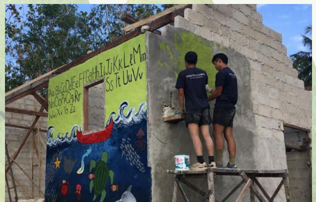
Building a play school in Bali as part of the Youth Expedition Project.
